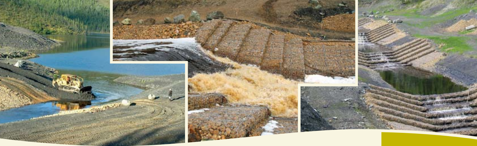
Photos from left to right: preparation for gabion baskets; gabion structure during spring run off and; gabion basket structures now in place
